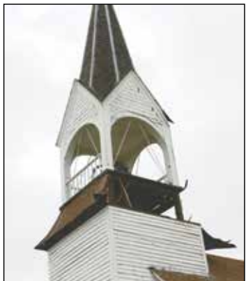
A section of the shingles were blown off by the storm.
