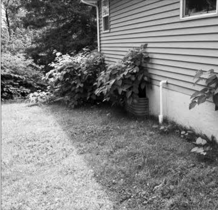
Knotweeds can grow into pavement and buildings which can require costly repairs.
