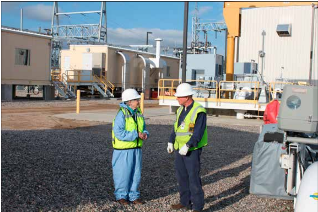
Mike Blowers, Engineer at Enbridge facility at Clearbrook answers questions for Mitzi Balstad of Fosston on the pump station tour that was held recently. Commissioners from Red Lake, Polk and Hubbard Counties and other interested persons were given a guided tour of the Enbridge pump station at Clearbrook. They were able to see how Enbridge's pipeline system serves as a vital link to stable and reliable North American crude oil supplies for Minnesota and the surrounding region.
